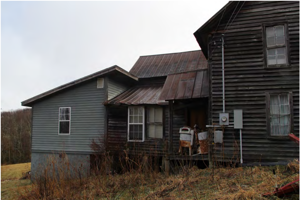
Nathan Hicks House, rear ell and addition, west elevation, view to east
